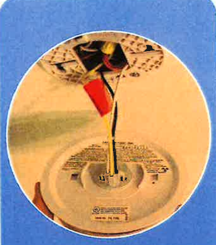
HARD- WIRED CARBON MONOXIDE ALARM
